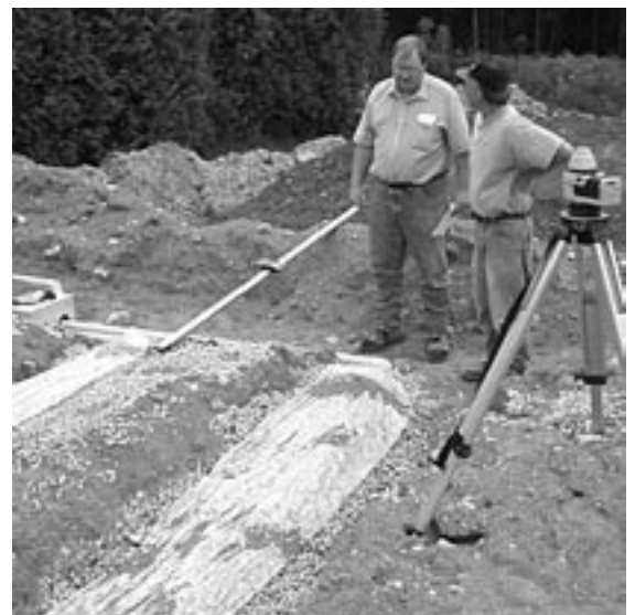
Inspection before being covered - the plastic on top helps prevent soil from filtering in and plugging the tile bed.
