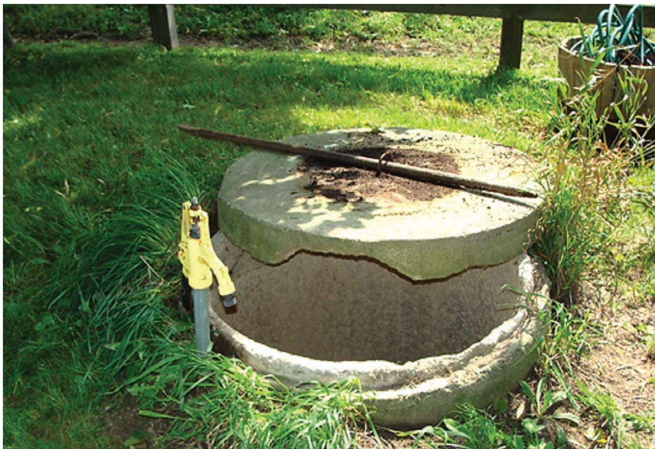
Figure 1: Damaged Lid and Casing
