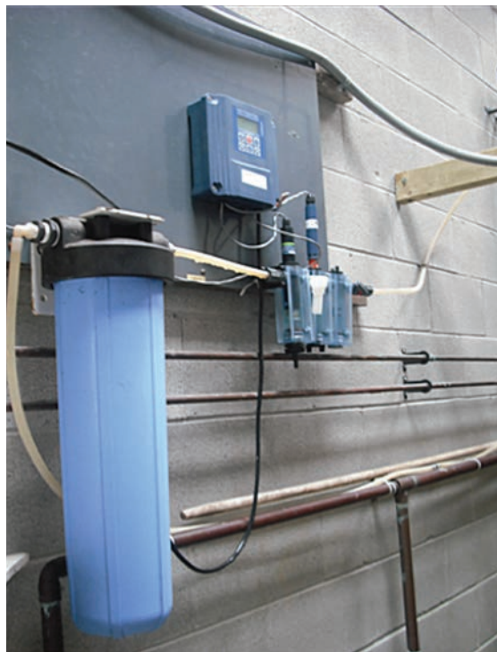
Figure 4: Chlorine and pH Monitoring System
